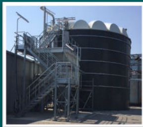
KLK Oleochemicals WWTP, Emmerich, Alemanha - 13 L/s
