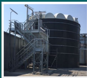
KLK Oleochemicals WWTP, Emmerich, Alemanha - 13 L/s
